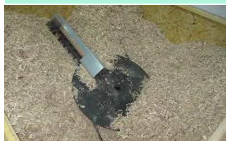
Wood chips storage (room) with the mixer connected to the transporter
